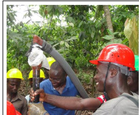
Figure 4. Swivel to allow rotation of the drilling rod without tangling the hose
